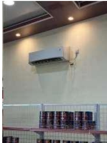
Figure 2. Steel and iron distribution building Air Conditioning System
