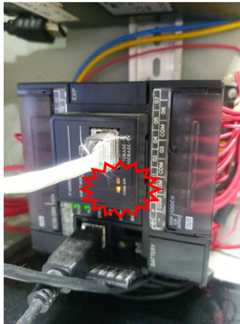
Figure 10. Indicator CP1W is already connected between PLC and HMI
