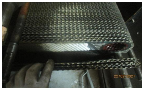
Figure 1. Salt Deposits On Evaporator
